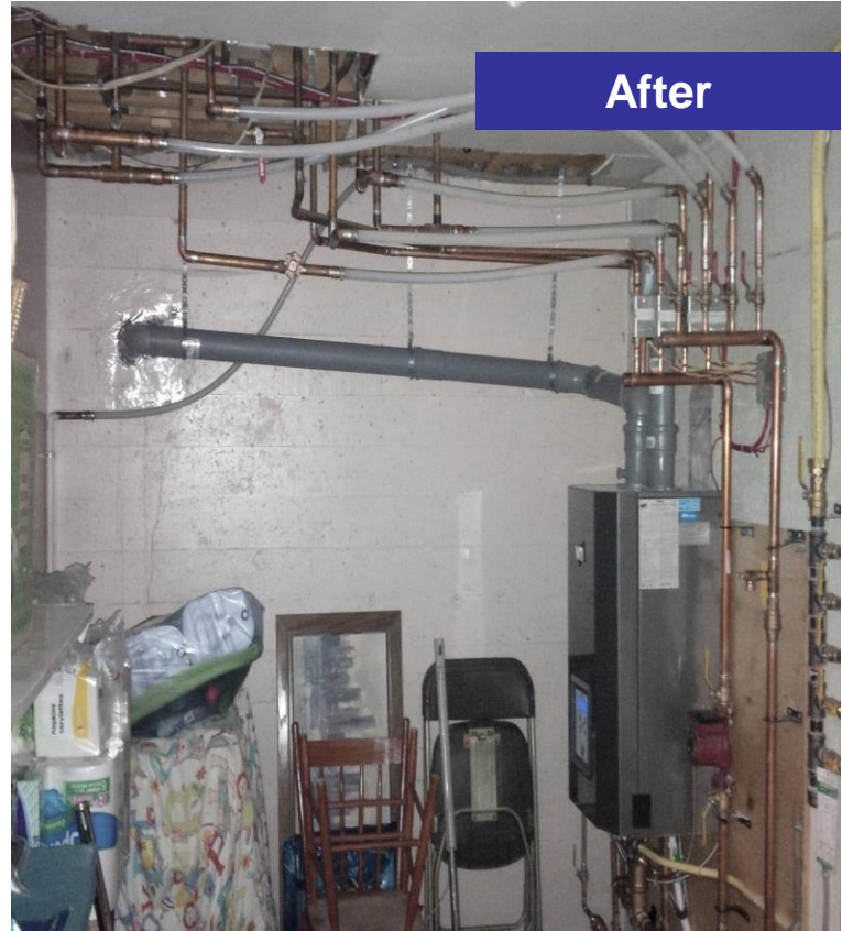
Propane boiler with tankless water heater built in
