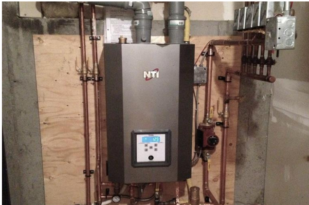
Propane boiler with tankless water heater built in
