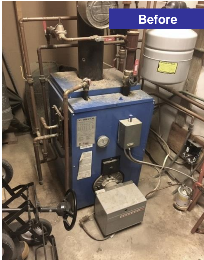
Oil boiler with coil
