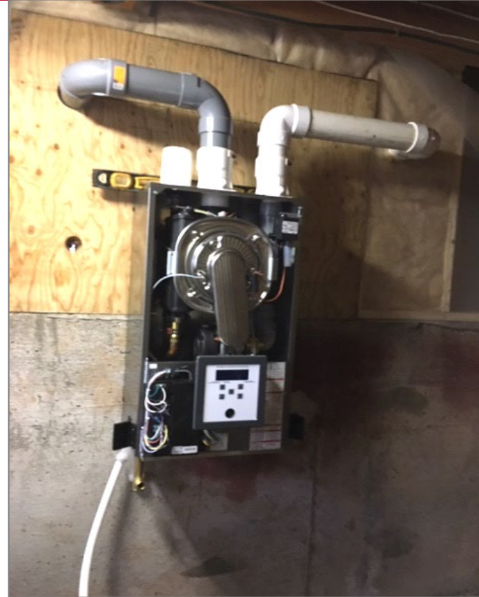
Propane boiler with tankless water heater built in
