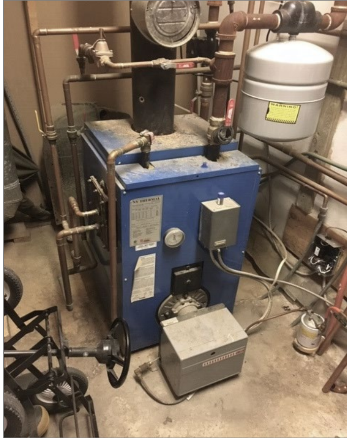
Oil boiler with coil
