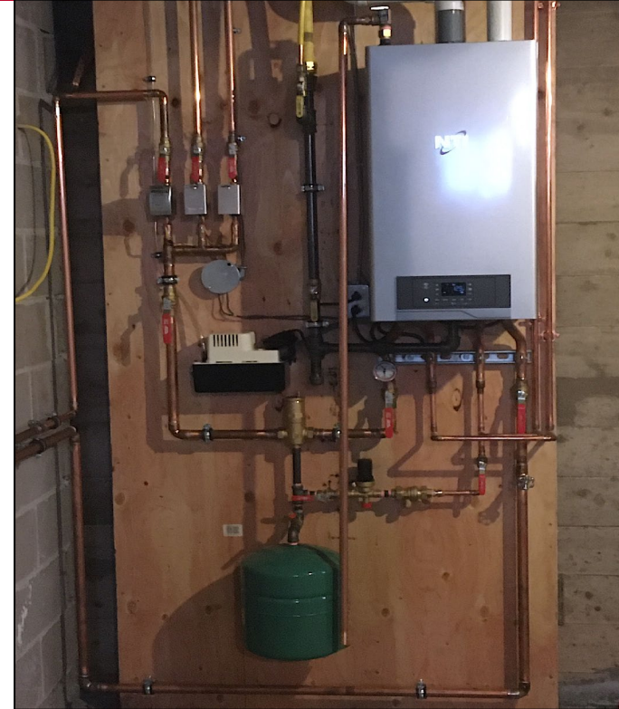
Propane boiler with tankless water heater built in
