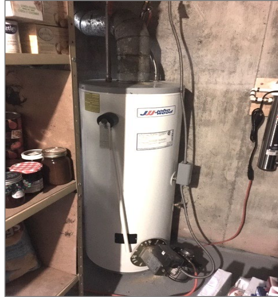
Oil water heater
