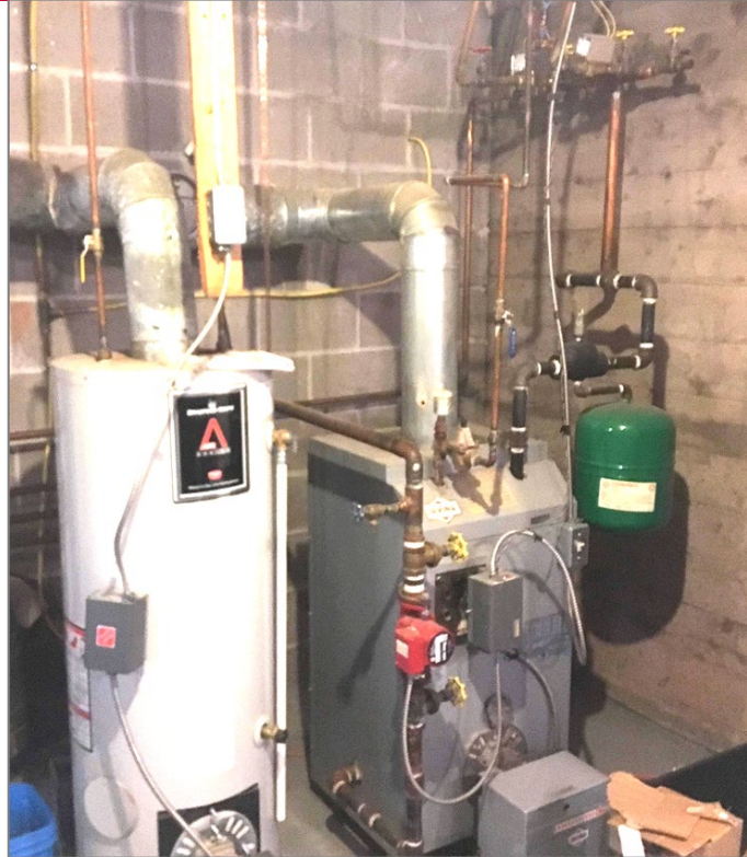
Oil boiler with oil water heater
