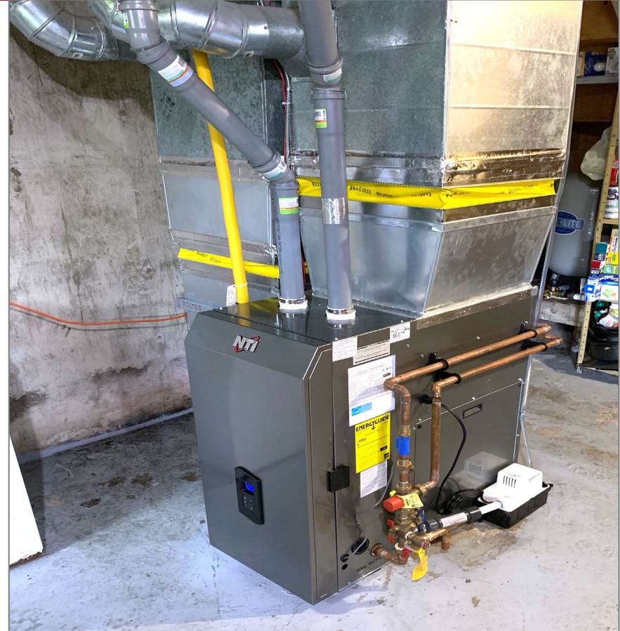
Propane furnace with tankless water heater
