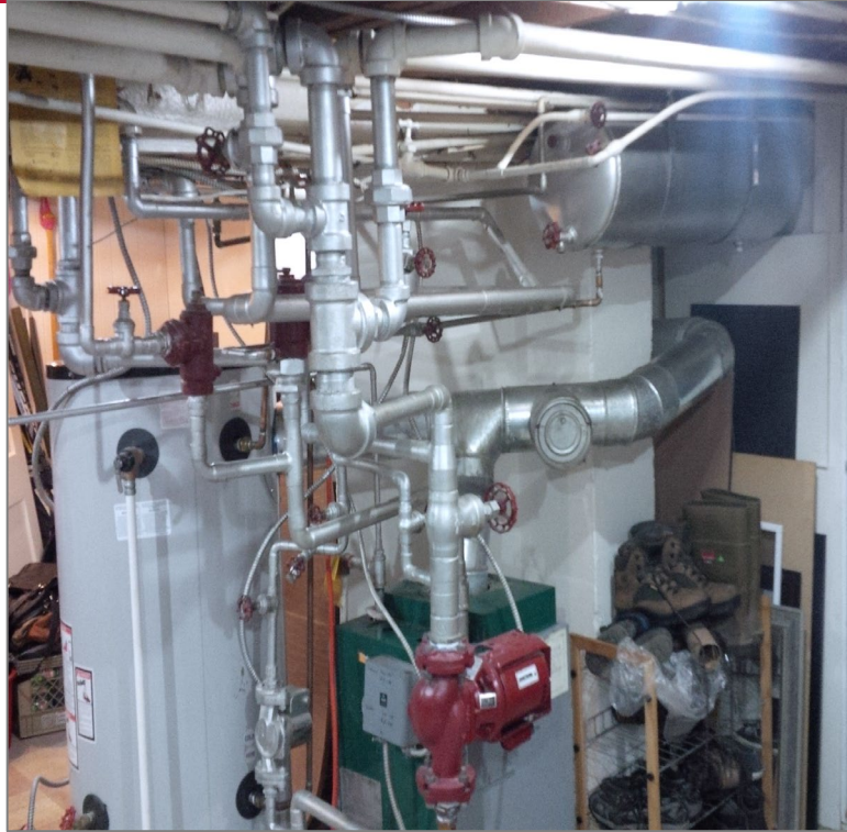
Oil boiler with electric water heater
