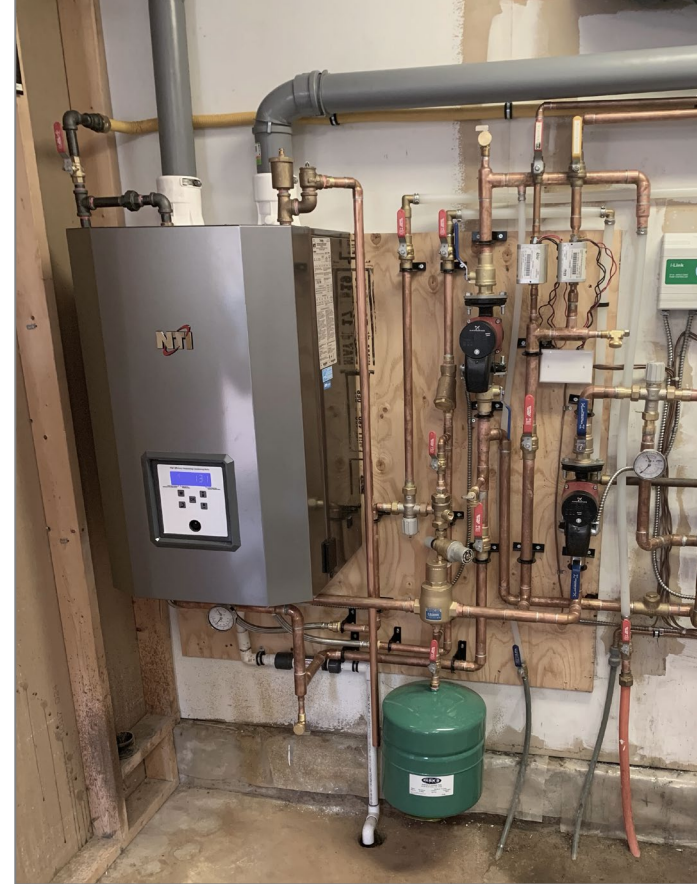
Propane boiler with tankless water heater built in
