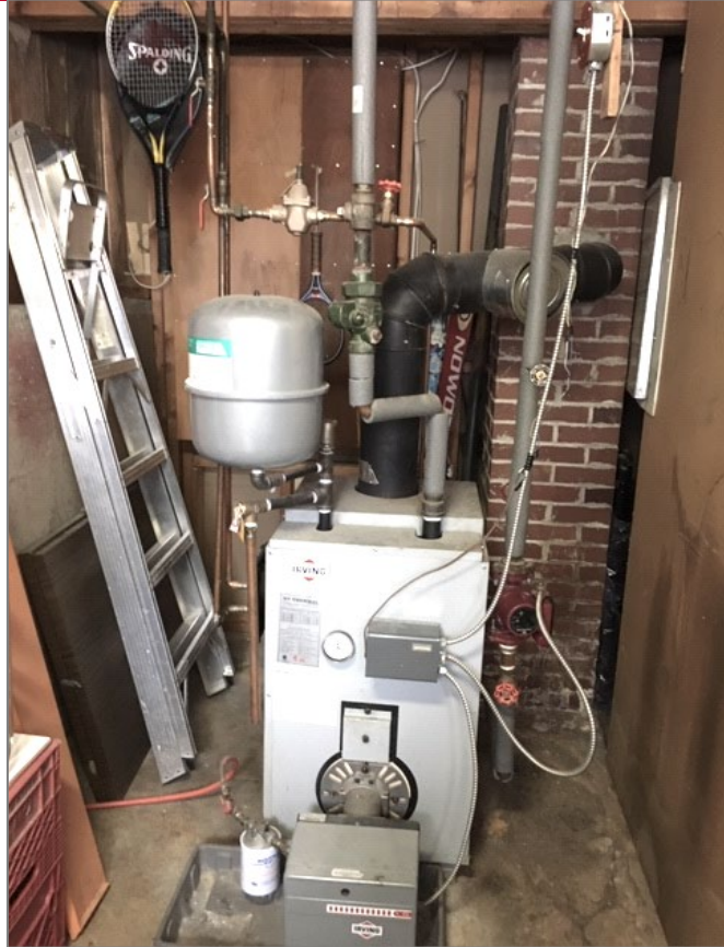
Oil boiler with coil
